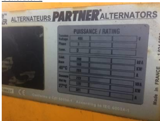
Fig1: Name Plate for 200 kVA Diesel Generator 1, JECO Power Station
