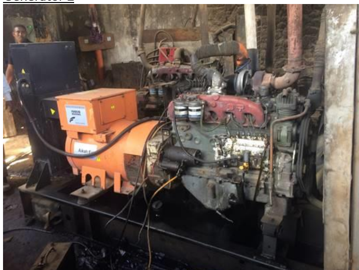
Fig2: 160 kVA Diesel Generator,
