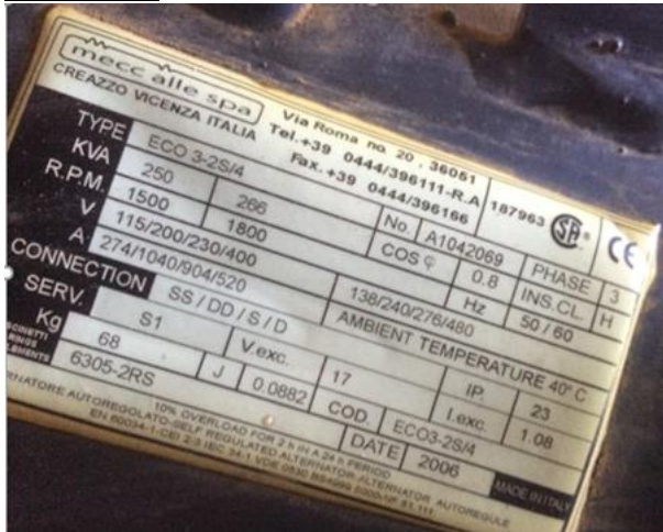
Fig4: Name Plate for 250 kVA Diesel Generator (faulted), JECO Power Station
