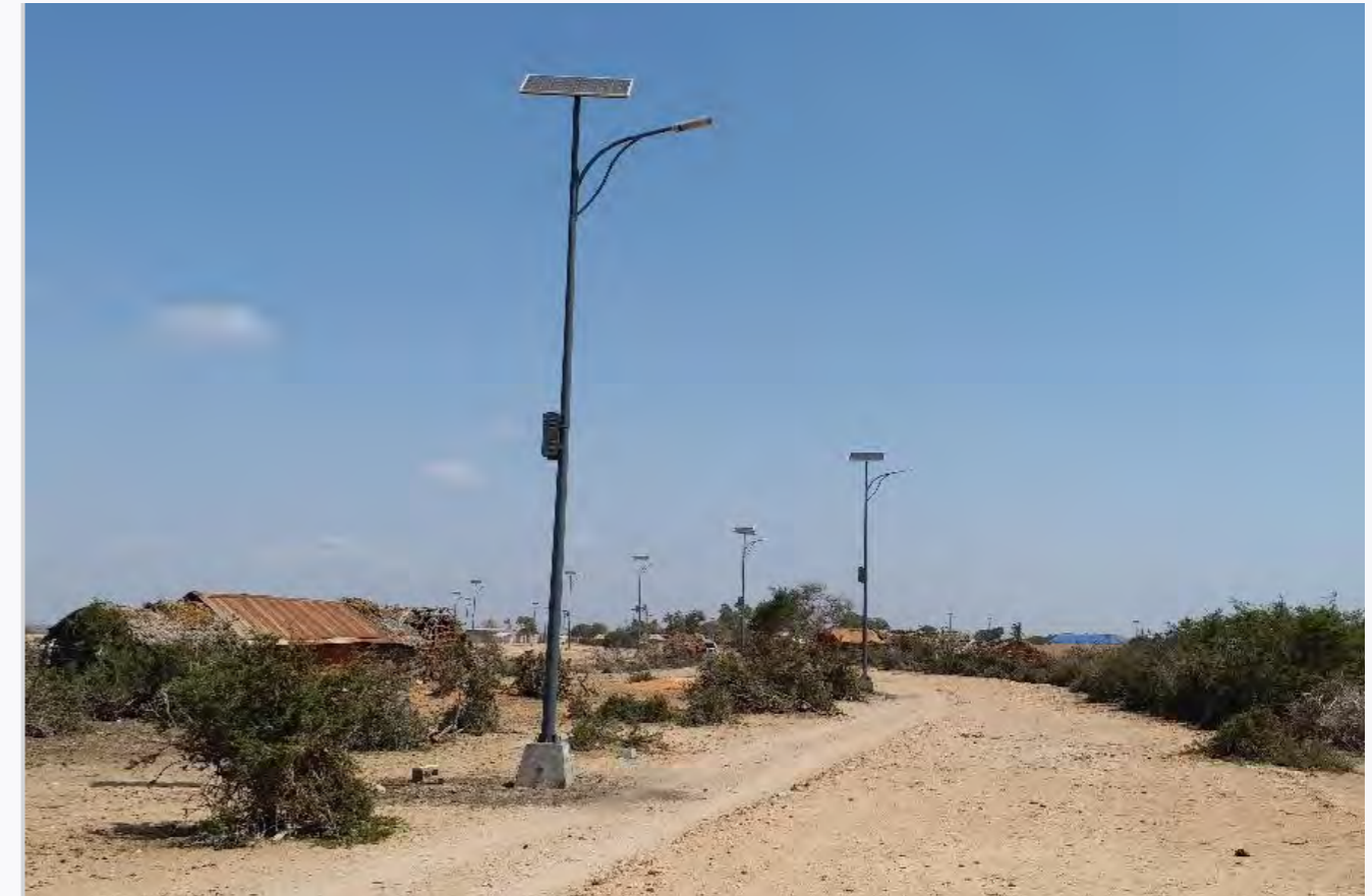
A total of 40 solar street lights were installed in the village of Gobweyn, Somalia.
