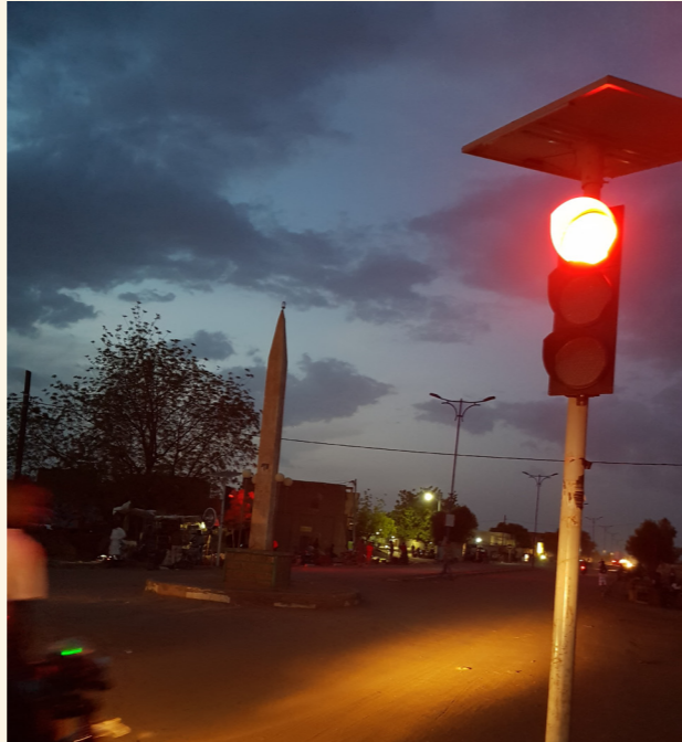
Photo: NIS. Solar traffic lights in Gao, Mali
