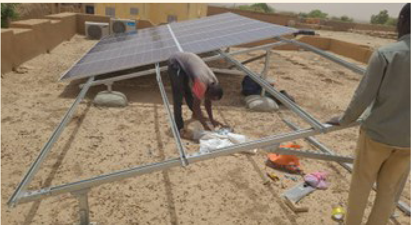
Photo: NIS. solar lights, Forgho, Mali
