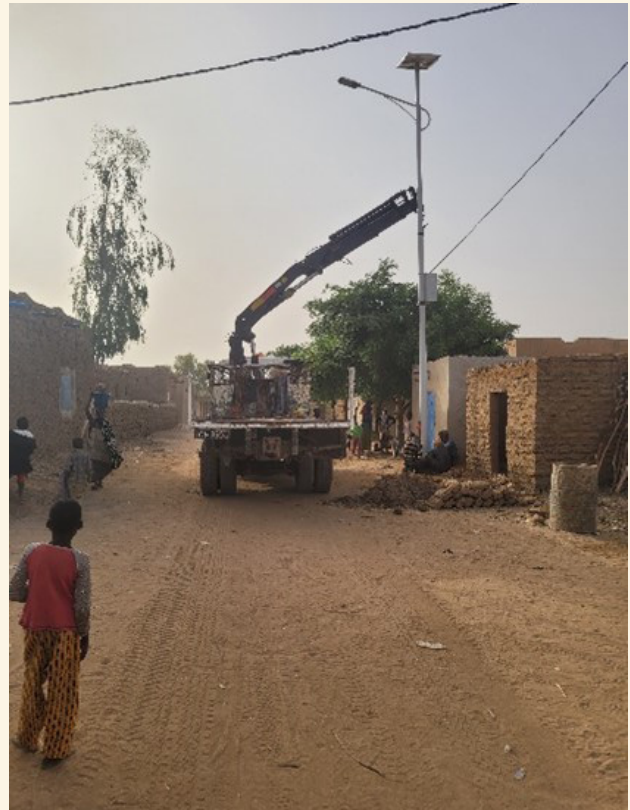
Photo: NIS. Solar panels, Bagoundje, Mali
