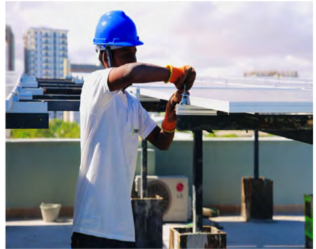
Mohamed Ise Osman working on solar installation with the Tamarso company. Photo by Hani Mohamed
