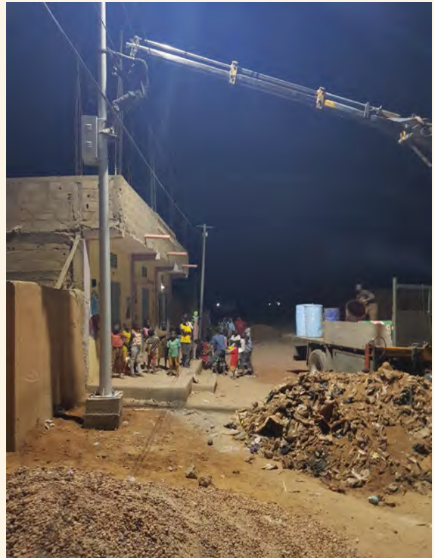
Photo: NIS. Solar Street Lights, Gao, Mali
